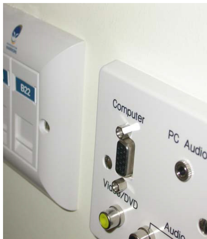
Thirty separate audio visual face plates for local connection to televisions in the hospitality boxes and other public areas.
